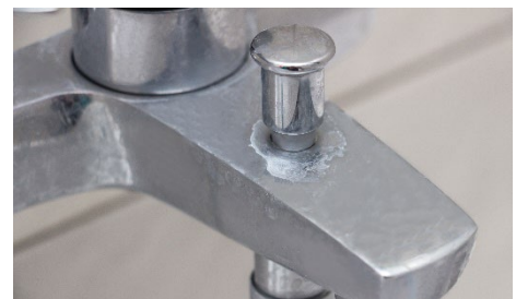
Mineral scale on water faucet
